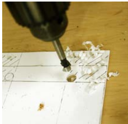
Figure 5-84. By drilling holes at any location where two bends intersect, you reduce the risk of the plastic fissuring.
